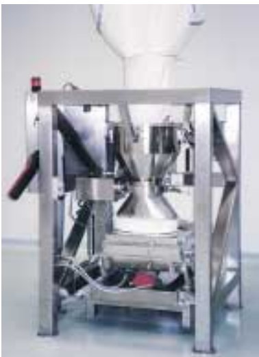
VDS, installed in a discharge station for super sacks
